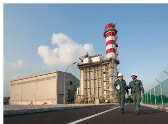
Commenced operation of the 400-megawatt Sembcorp Cogen @ Banyan in October, strengthening our market leadership on Jurong Island, Singapore
