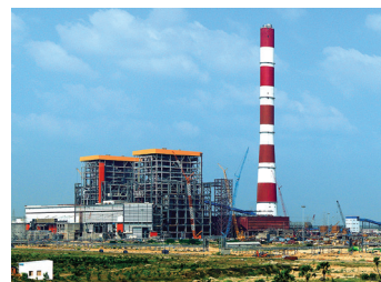
Marked a milestone at our first power project in India, Thermal Powertech Corporation India, with the synchronisation of the plant's first 660-megawatt unit to the grid
